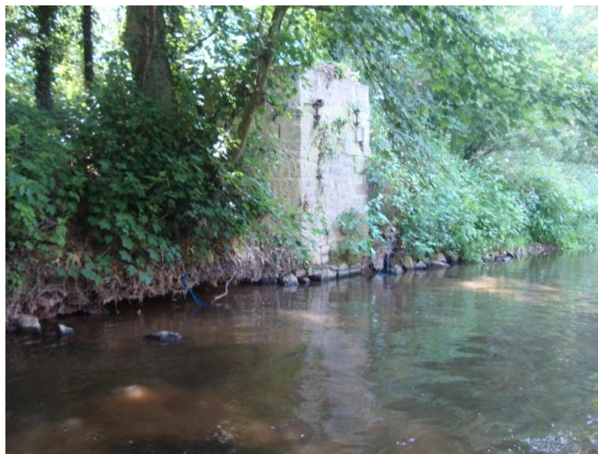
Plate 7. The blockwork foundations located upstream of Site 2 entrance that were under construction to provide a footbridge over the river.
