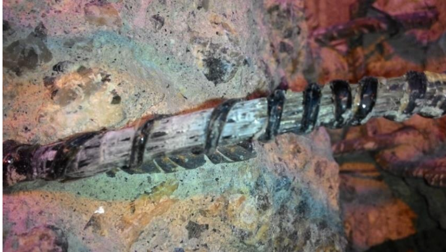
Photo 8: Basalt B2: basalt spiral strands are debonding from longitudinal strands.
