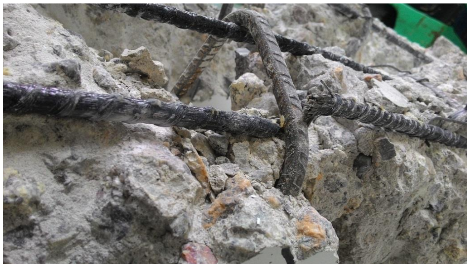
Photo 12: Beam B3 Reinforcement Failure.
