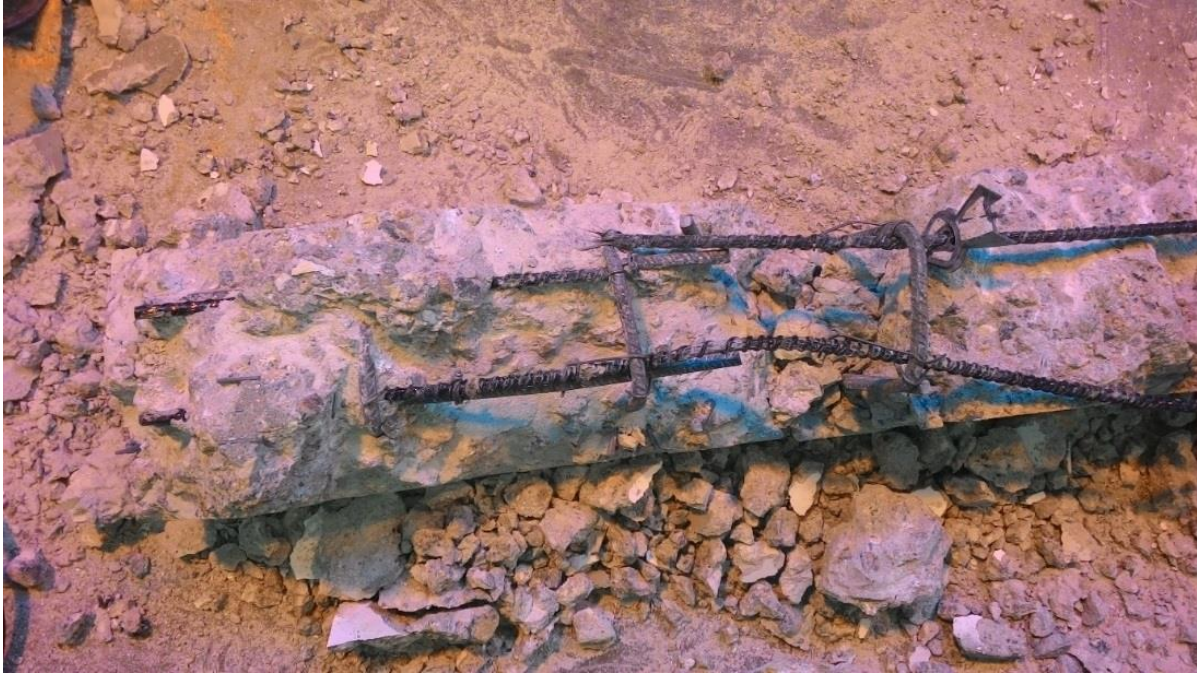
Photo 10: Basalt B2: bottom face of the beam.
