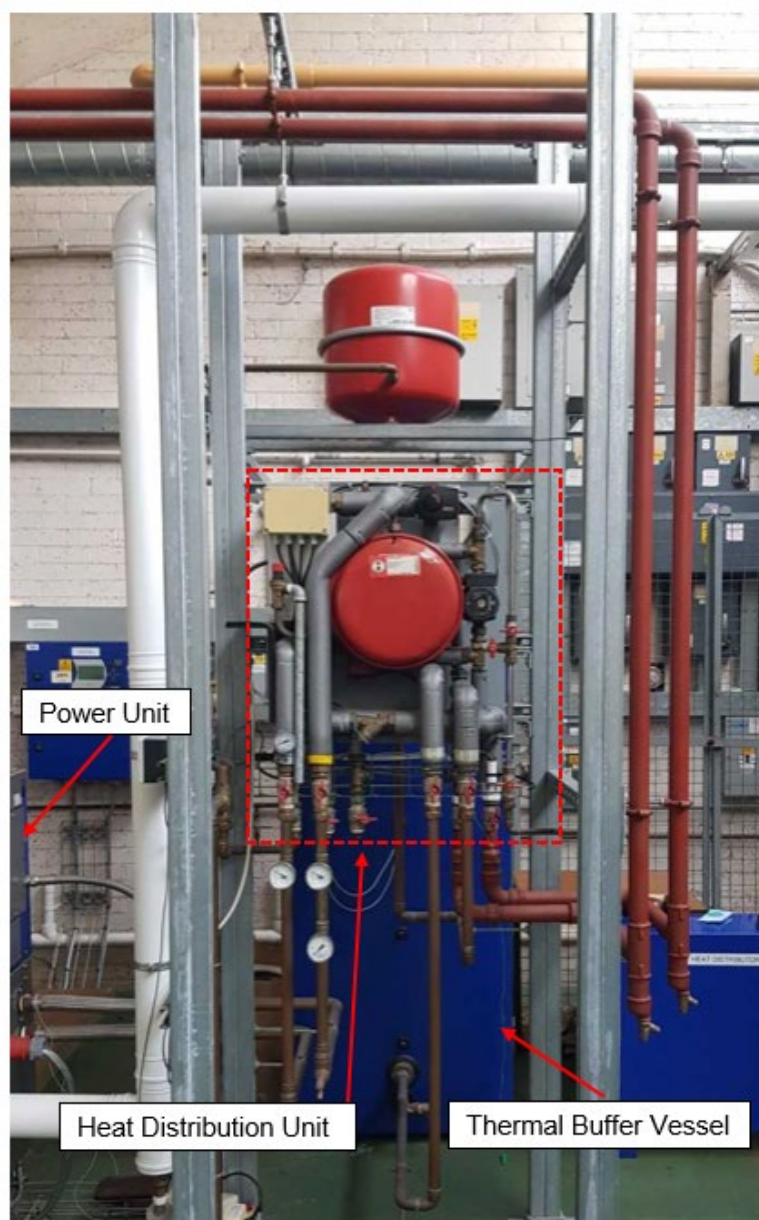
Figure 2: Heat Distribution Unit and Buffer Vessel
