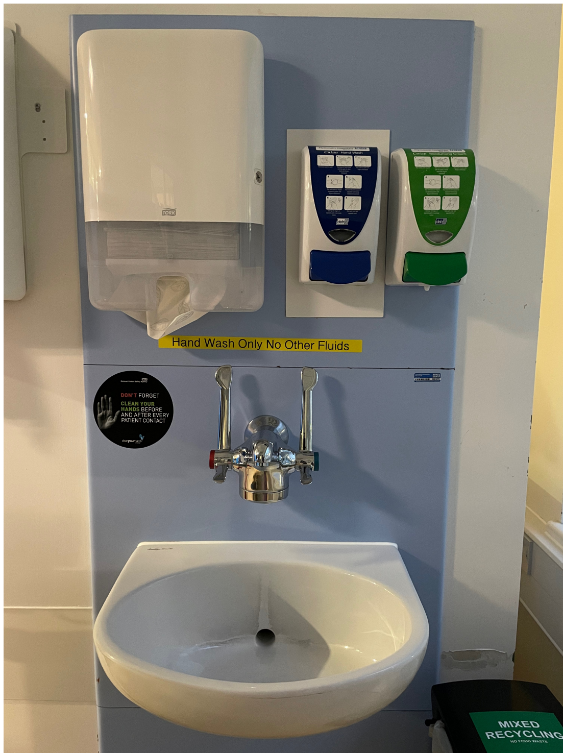
Figure 1.3: Sink on a high-dependency ward of Derriford Hospital (University Hospitals Plymouth NHS Trust) showing a sign indicating that the sink should be used for handwashing only, suggesting increased awareness that the use of ward sinks for disposal of fluids other than in handwashing is problematic. Picture taken in December 2021.
